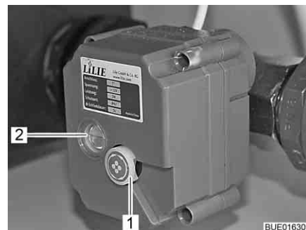
Fig. 212 Electrically operated drainage valve
