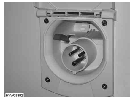
Fig. 141 230 V connection on vehicle
