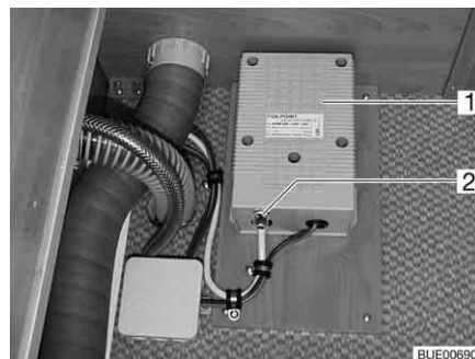
Fig. 152 Transformer for electrical floor warming unit
