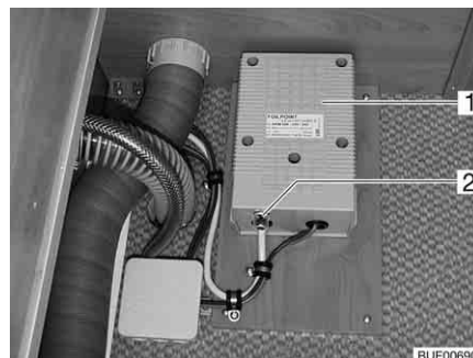
Fig. 197 Transformer for electrical floor warming unit
