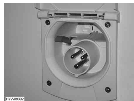
Fig. 168 230 V connection on vehicle
