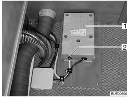
Fig. 144 Transformer for electrical floor warming unit
