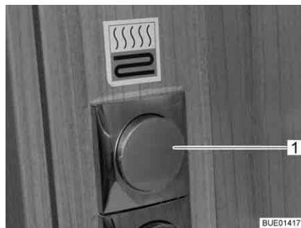
Fig. 119 Switch for floor warming unit in toilet compartment
