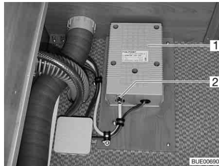
Fig. 117 Transformer for electrical floor warming unit
