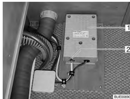
Fig. 123 Transformer for electrical floor warming unit
