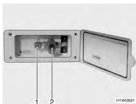
Fig. 91 External gas connection, gas isolator tap closed
