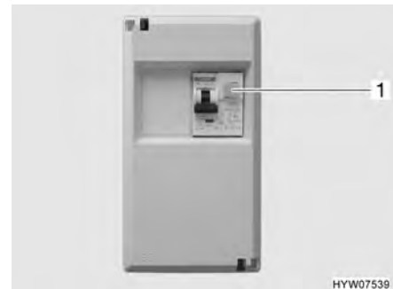
Fig. 105 230 V fuse box with safety cut-out and fault current protection switch (FI)
