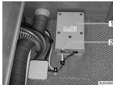
Fig. 195 Transformer for electrical floor warming unit
