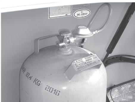
Fig. 75: Pressure reducing valve
