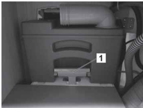
Fig. 203: Waste holding tank in the disposal shaft
