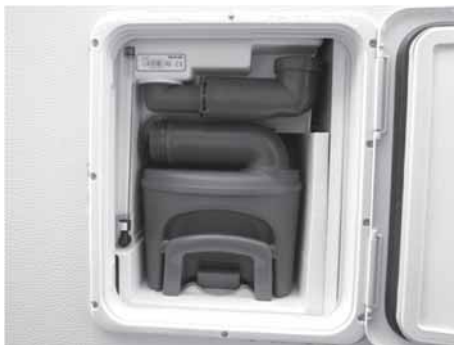
Fig. 46: Holding tank with flushing water intake port
