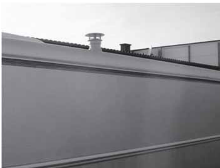
Fig. 82: Exhaust gas stack of the gas heater
