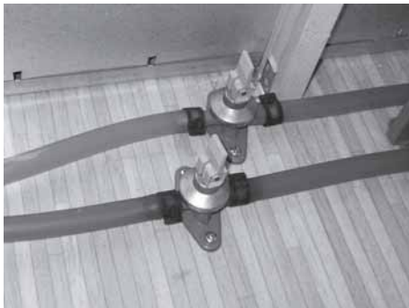
Fig. 102: Drain valves opened
