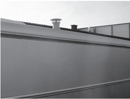
Fig. 83: Exhaust gas stack of the gas heater
