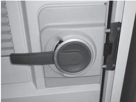
Fig. 13: Closed but unsecured door lock
