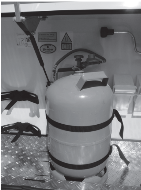
Fig. 74: Open gas locker
