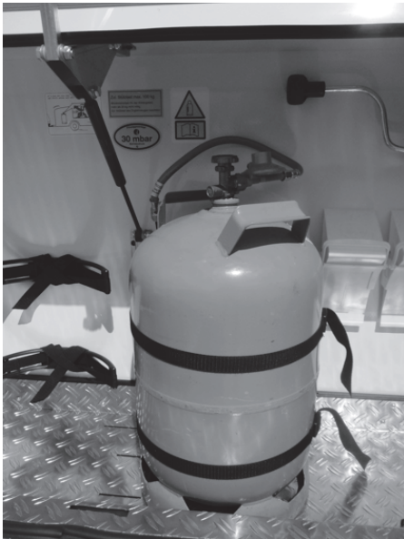
Fig. 75: Pressure reducing valve
