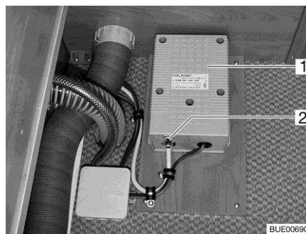
Fig. 168 Transformer for electrical floor warming unit
