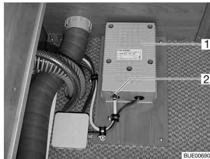
Fig. 205 Transformer for electrical floor warming unit
