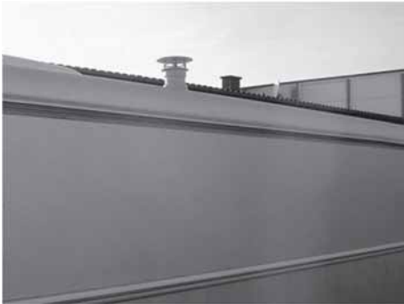
Fig. 74: Exhaust gas stack of the gas heater
