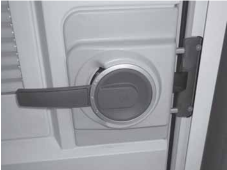
Fig. 13: Closed but unsecured door lock
