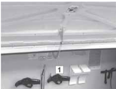
Fig. 68: Open gas locker
