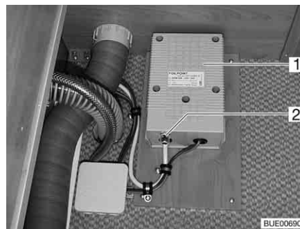
Fig. 152 Transformer for electrical floor warming unit
