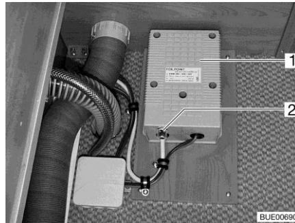
Fig. 224 Transformer for electrical floor warming unit
